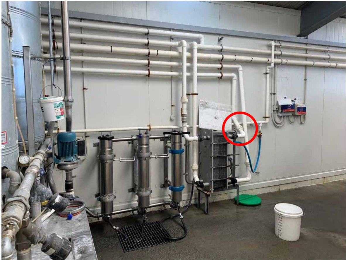
Figure 61 Example of a low flow tap next to milk filter in dairy shed
