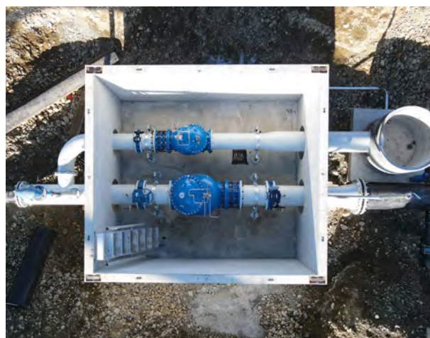
PRV 6 after upgrade
