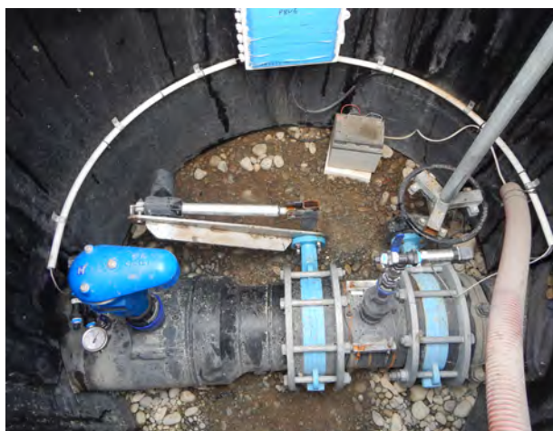
PRV 6 before upgrade
